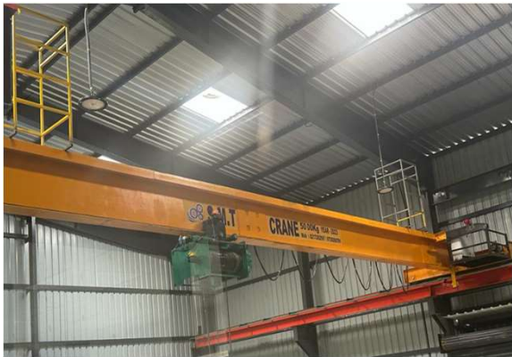
Overhead Crane 5T Capacity
